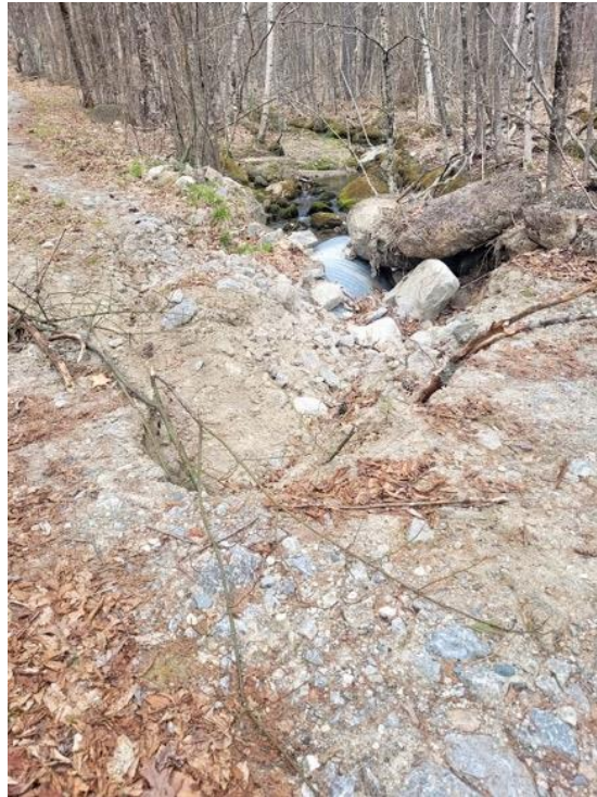
Washout noted in 2024
